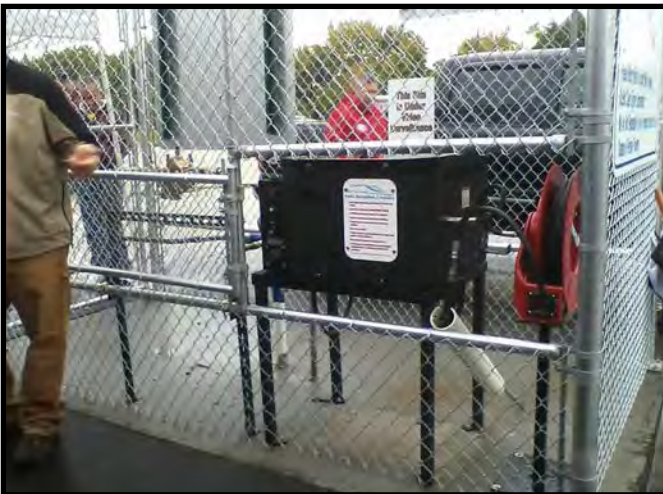
Self service coin-operated boat wash station in Lacrosse, WI
